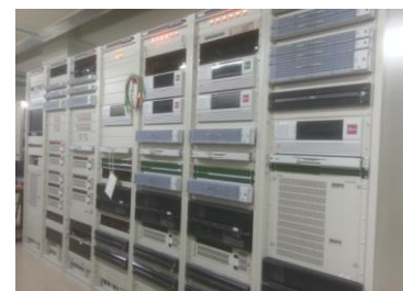
Photograph 3 – Part of the Transmission facilities
